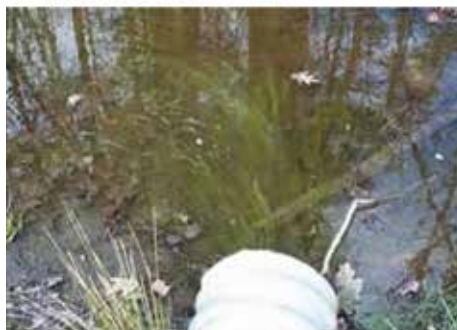
Strands of algae from a drainage pipe.
